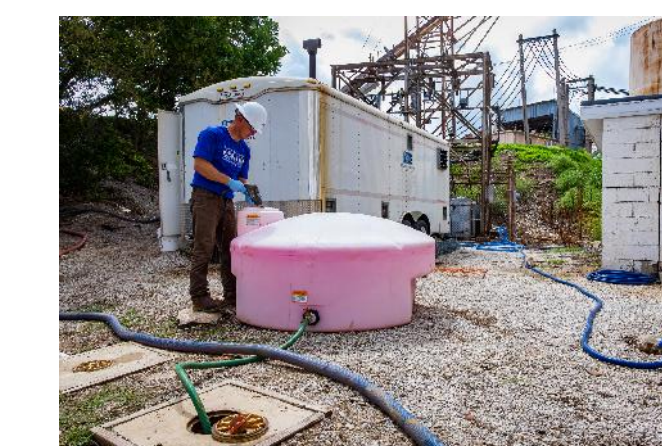
Surfactant, water and tracer dye were mixed at the surface and gravity fed into the targeted well.
